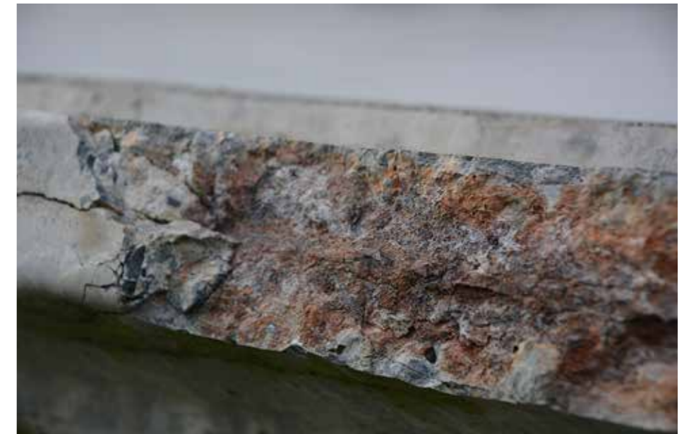
Corroded slat: strength is weakened and high risk of failure
